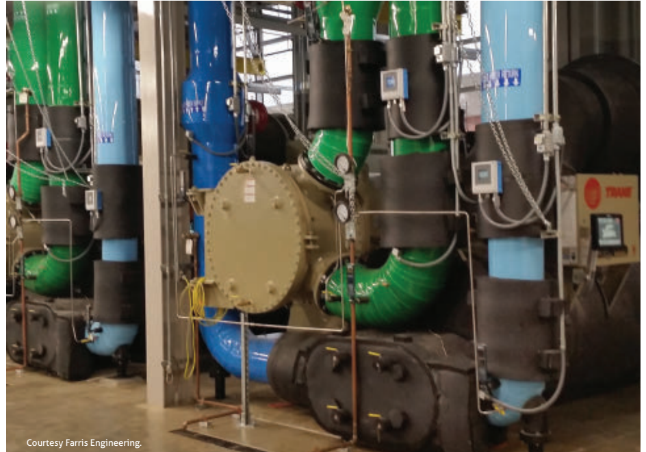
North Chiller Plant piping, South Dakota State University.
